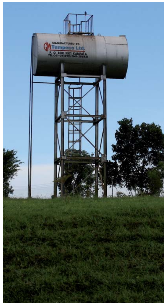
Water Storage Tank, Uganda
