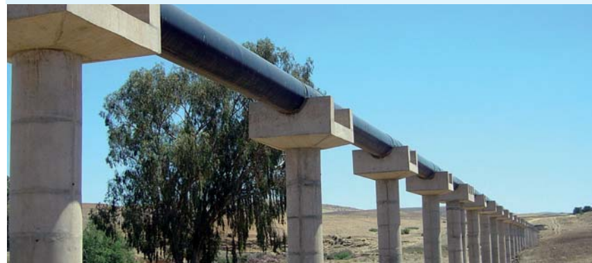
Water pipeline, Sidi Bel Abbès, Algeria
